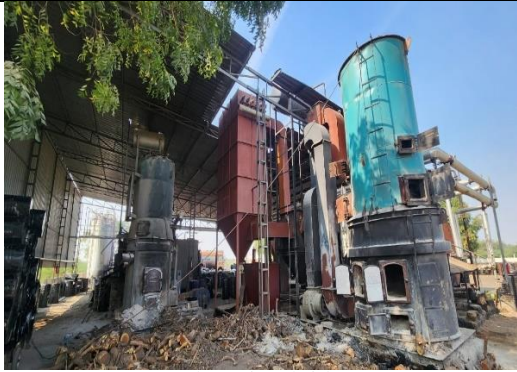
Thermic Fluid Heater
