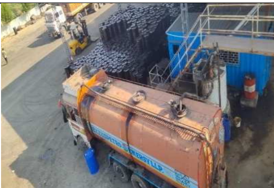
Emulsion Bitumen Loading Point
